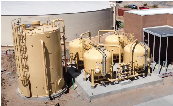
Airline Lambert Water Treatment Campus
