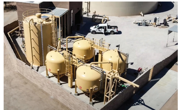
Picture Rocks Water Treatment Campus
